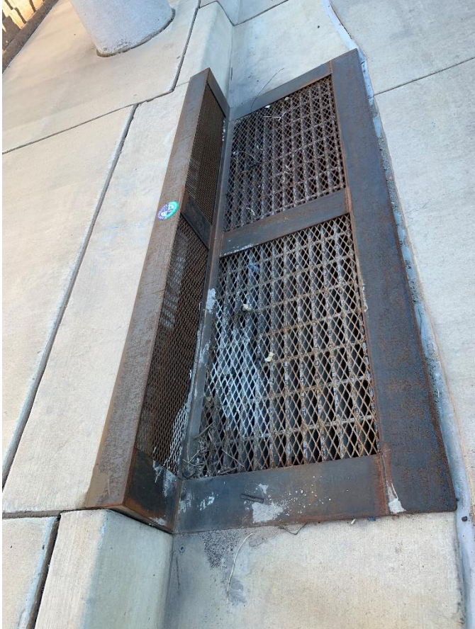
Mesh covering for storm drains
