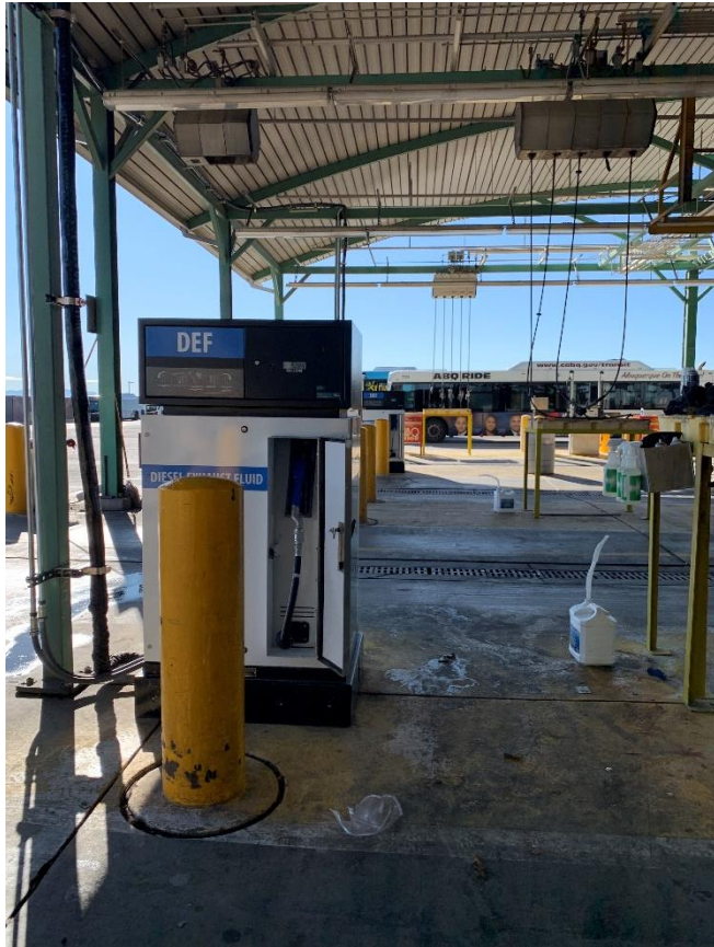
Diesel Exhaust Fuel (DEF) Pumps.
